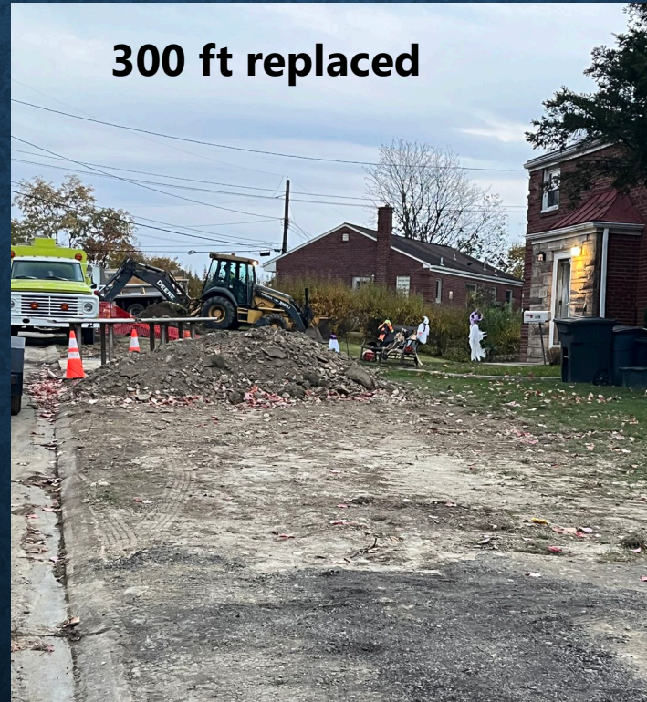
Klementina Water Line
